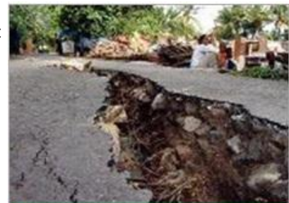
DAMAGE FROM THE 6.9 MAGNITUDE EARTHQUAKE IN CEBU
